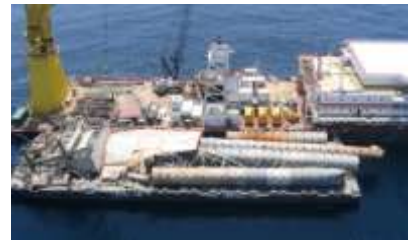
1,876 tons of salvaged components secured on 250' material barge for transport and onshore disposal.
